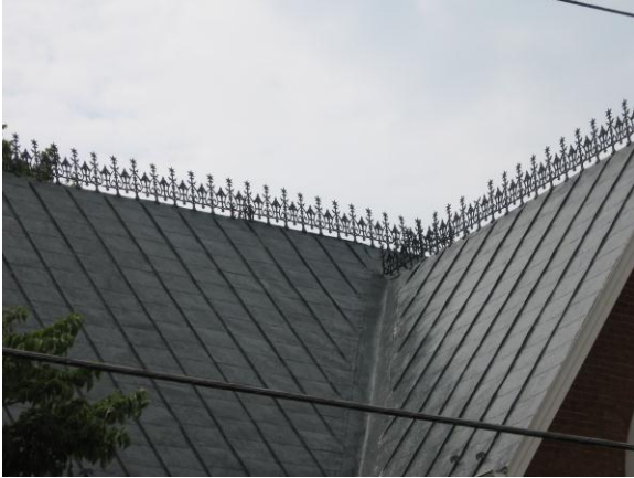
Original metal standing seam roofs should be maintained and repaired if needed (602 Washington Street).
