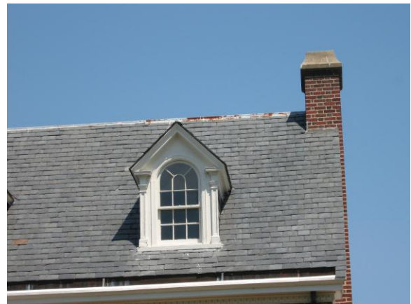
Roof features such as dormers should be preserved and maintained (3104 Rivermont Avenue).
