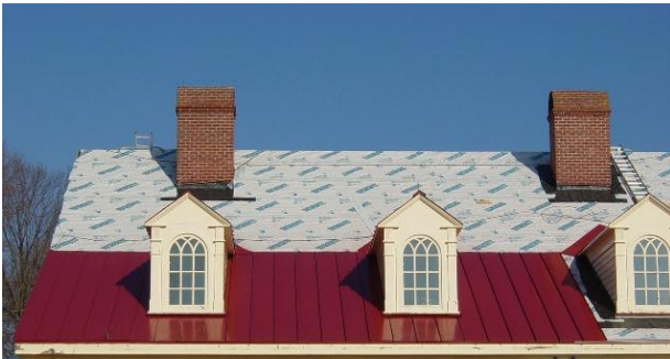
If replacement is necessary use a metal seam roof similar in dimensions, spacing and crimping as the original.
